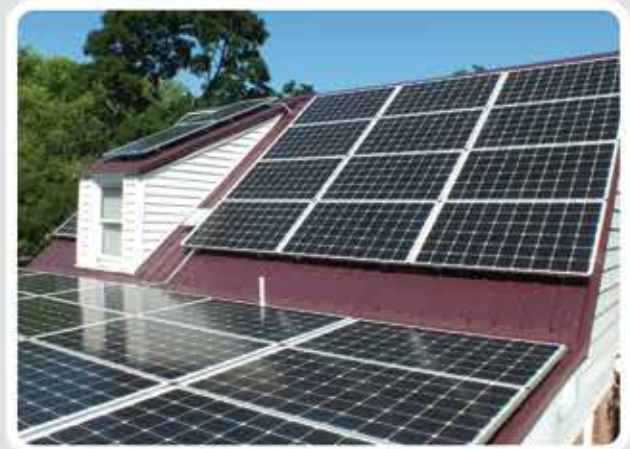
SOLAR POWER SYSTEM
