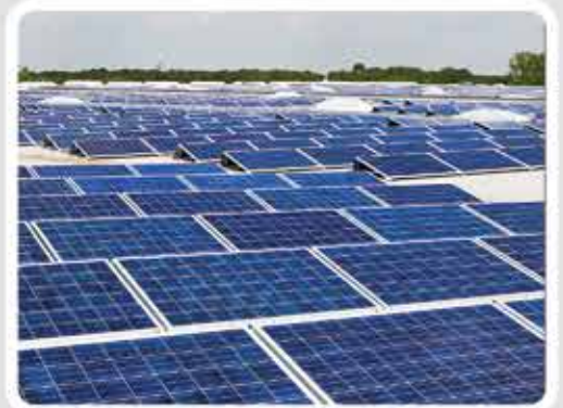
SOLAR POWER SYSTEM
